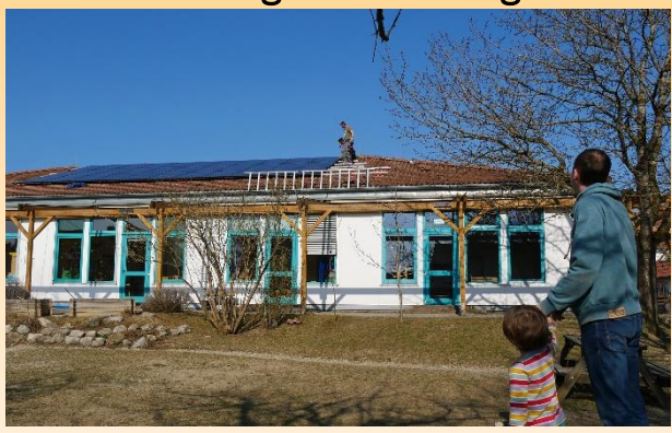
Photovoltaik-Dachanlagen Kindergarten Mering
